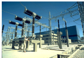
High Voltage Sub-Stations
