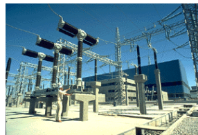
High Voltage Sub-Stations
