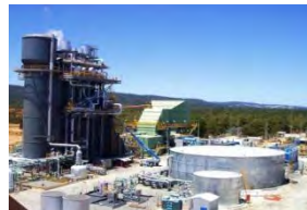
Natural Gas Fired Co-generation Plants
